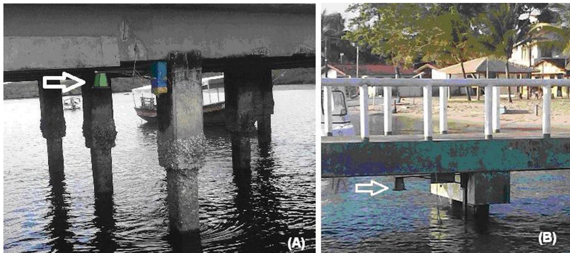
FIGURE 7. TidalDuino system installed under the piers of (A) Ituberá and the (B) Barra do Serinhaém.
